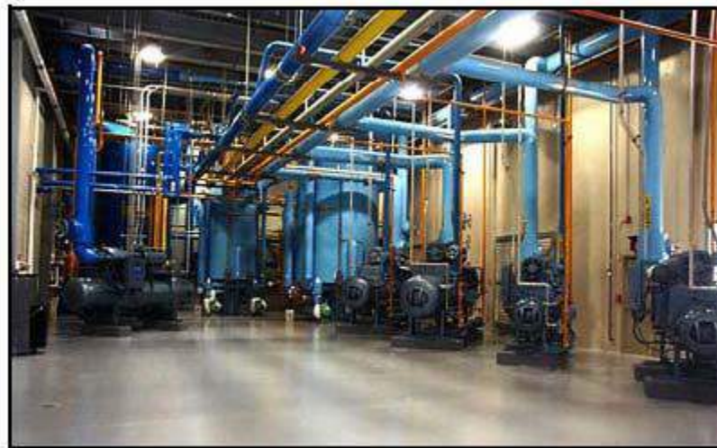
Fig.1.10 Ammonia based refrigeration plant for a large cold storage
